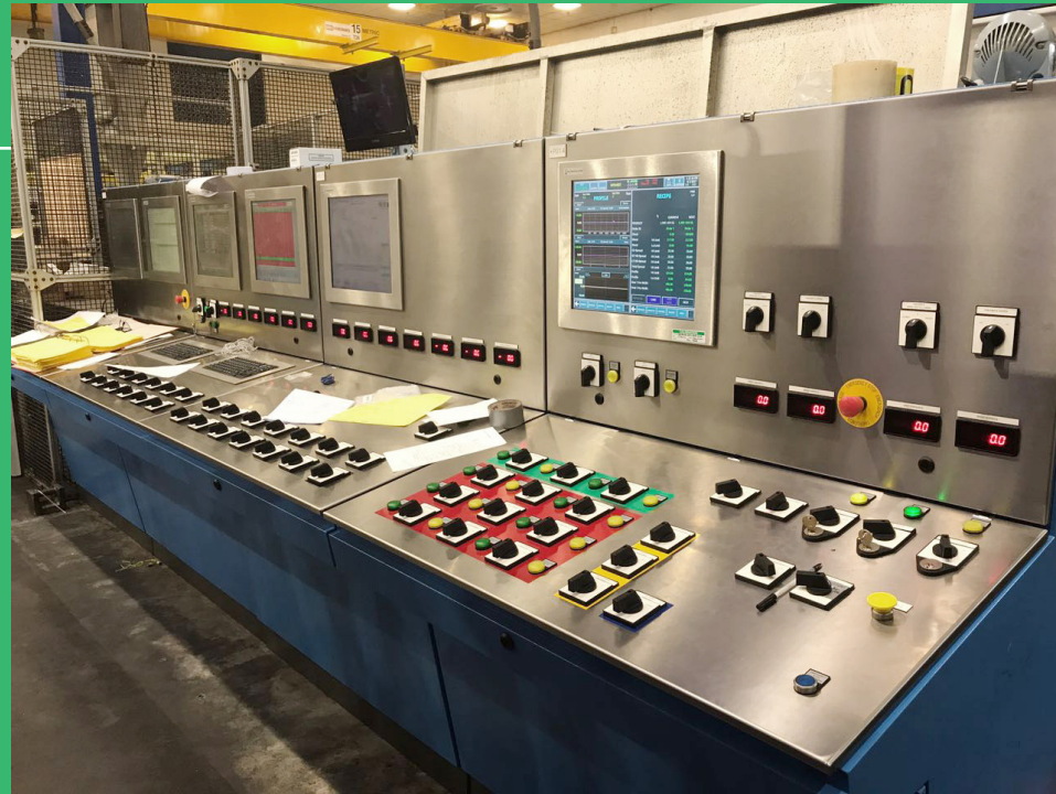
New main control panel
